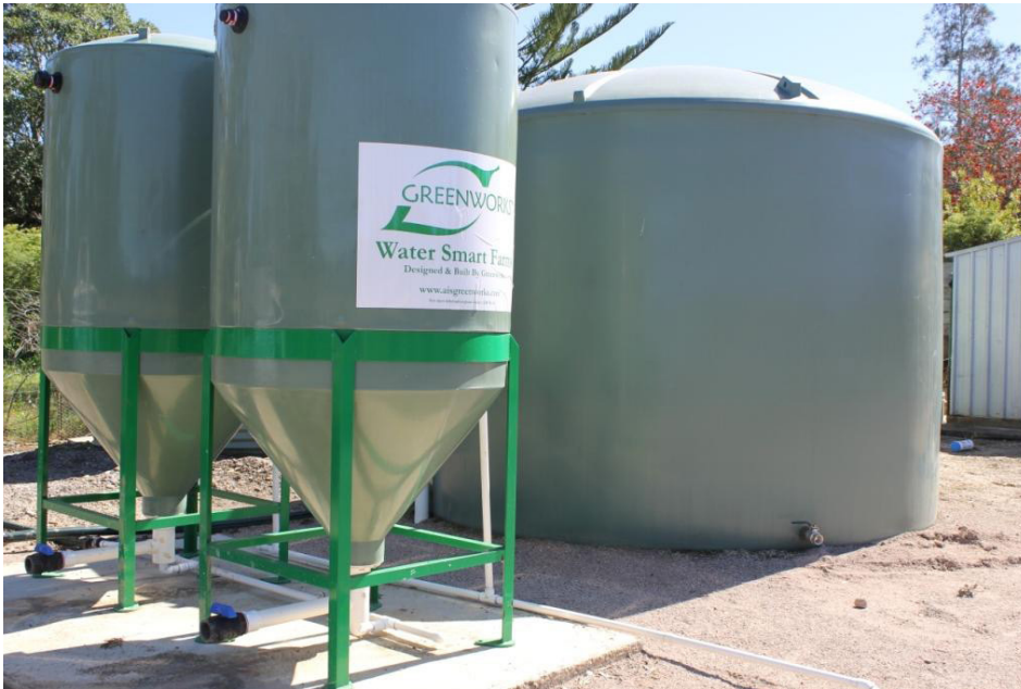
Water treatment, collection and recycling at Cameron's Nursery, NSW.
