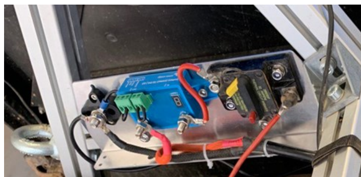
Figure 2. Circuit breaker with yellow and red buttons.
