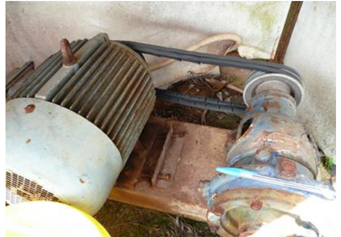
Figure 2: Old belt drive irrigation pump sitting on ground, never serviced and in poor condition, pumping efficiency < 30%
