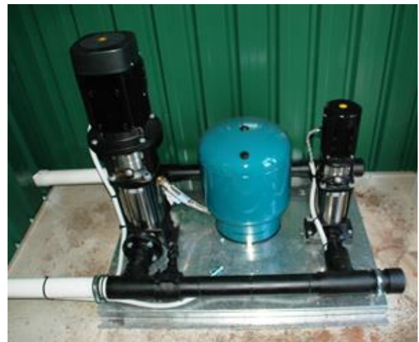
Figure 3: New twin pump set combining a small and large pump to provide various pressures
