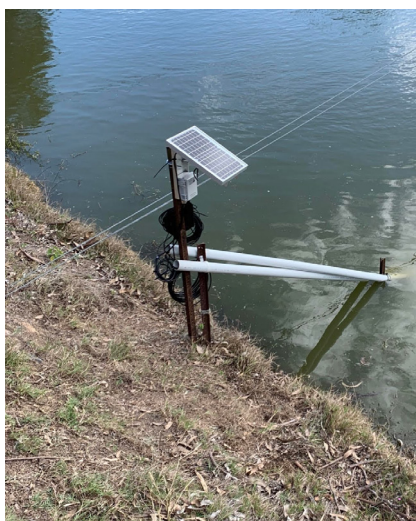
Dam temperature, pH, EC, REDOX and salinity monitoring
