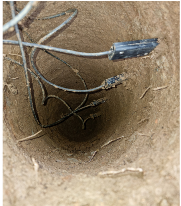
Soil moisture sensors installed 10, 20, 40, 60, 80cm
